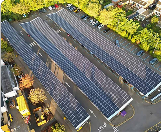
FIGURE 5.4 Hull University Teaching Hospital's solar carport canopy
